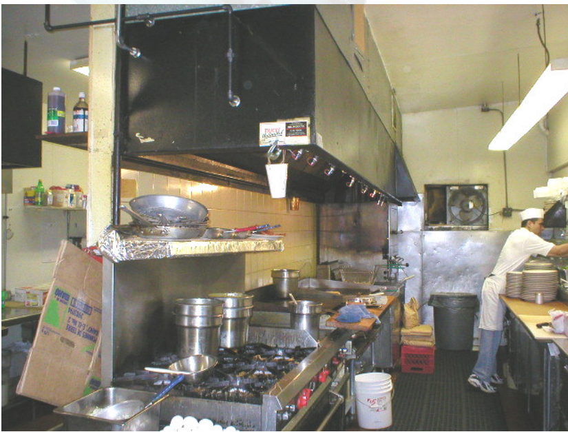
Kitchen – Main Line
